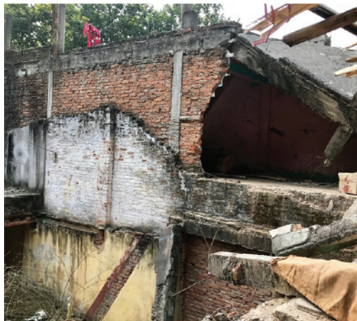
Damage seen near the epicenter in February 2020
