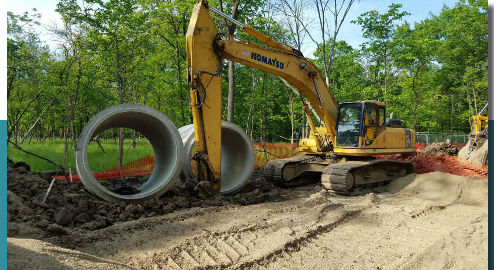
Cleveland Stormwater Separation Project in collaboration with Metropolitan Reclamation District, the IEPA Revolving Loan Program, and the Cook County Forest Preserve District
