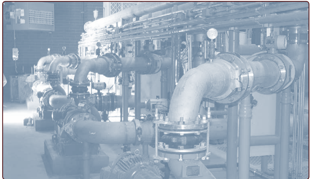
These projects are the basic building blocks of our economy — water and wastewater treatment plants (Alamosa's shown above), water and sewer mains, street expansion and resurfacing, affordable housing and community development. Photo by Richard P. Arber Associates.
