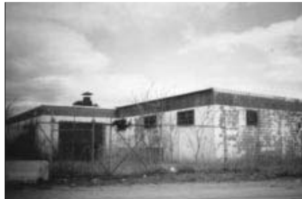
Redeveloping abandoned and deteriorating structures is a priority for the city of Bridgeport.
