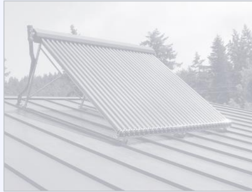
Solar Hot Water
