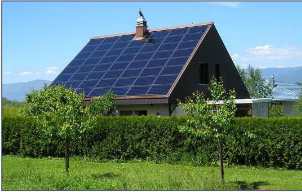
Solar Photovoltaic (PV)
