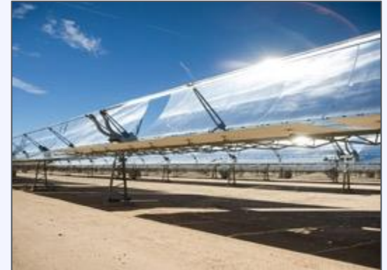
Concentrated Solar Power
