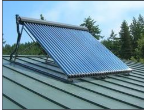
Solar Hot Water
