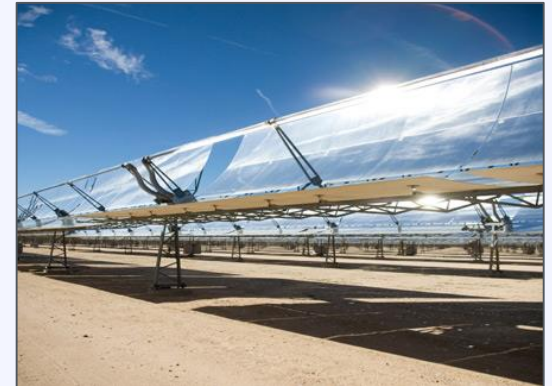
Concentrated Solar Power
