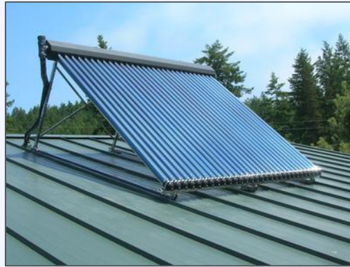
Solar Hot Water
