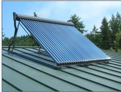
Solar Hot Water
