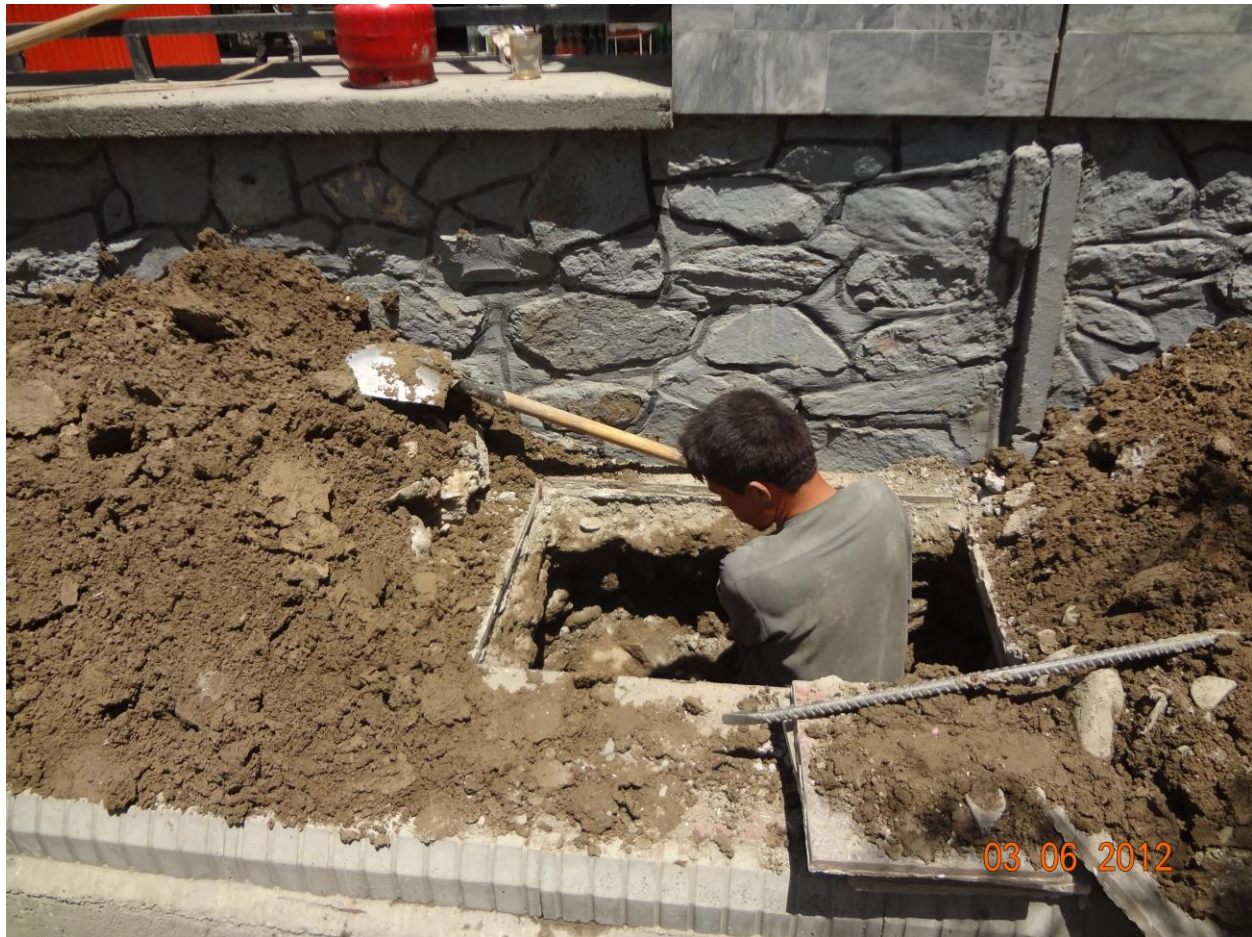
Preparing to lay the fiber optic cable for a higher speed internet connection at MAIL.
