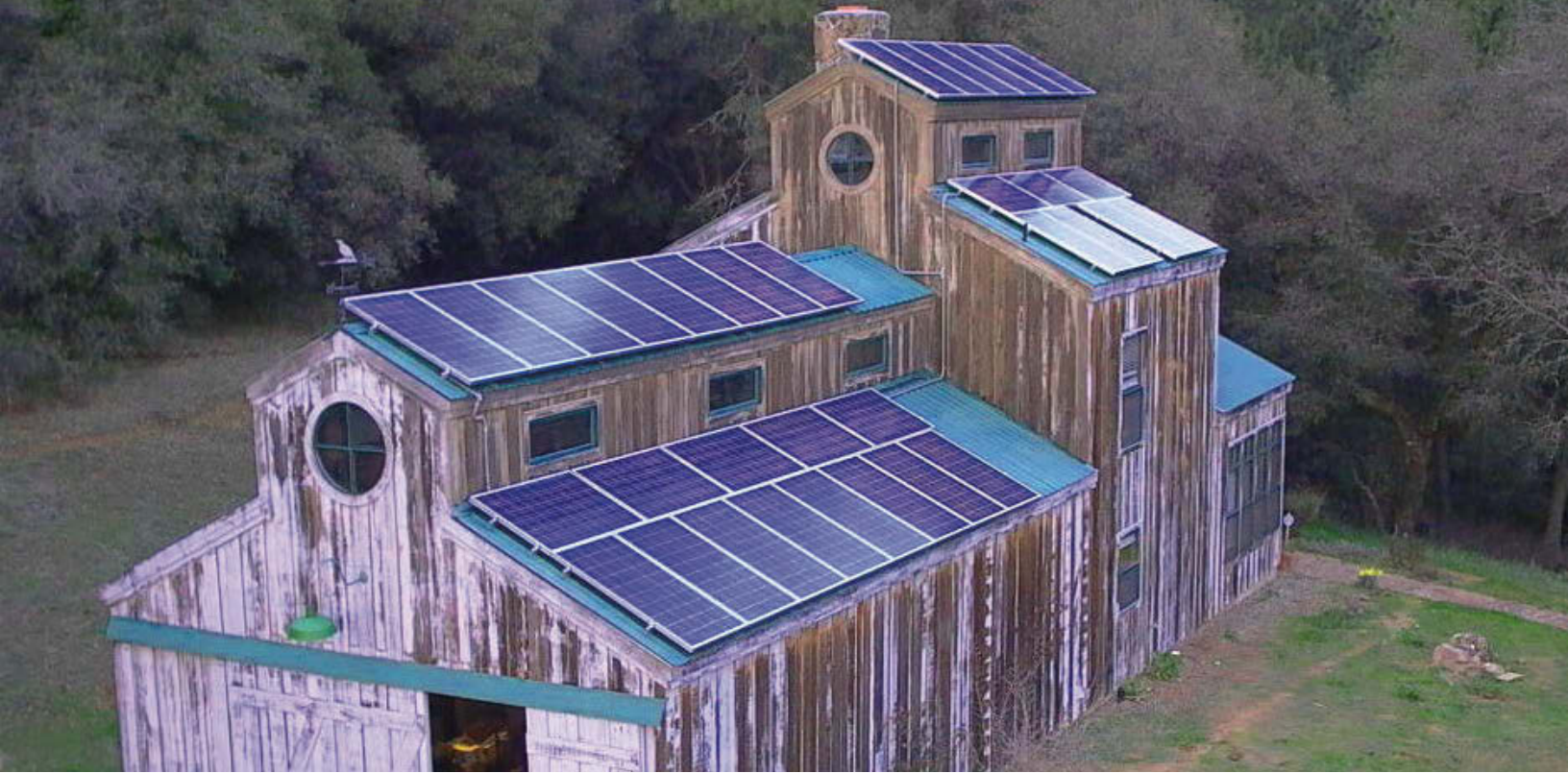
Rural PV installation in Colorado
