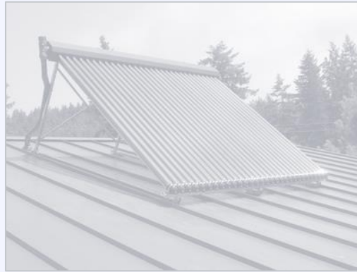
Solar Hot Water
