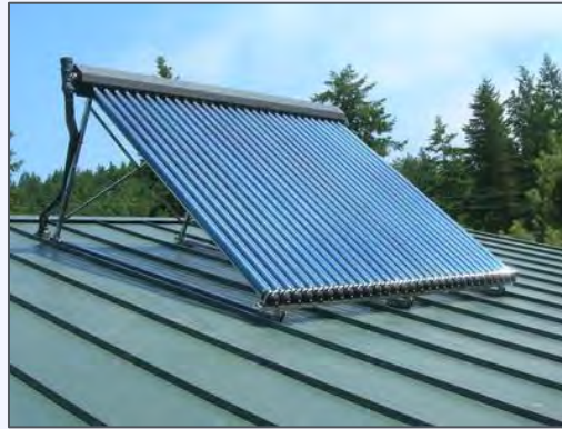
Solar Hot Water
