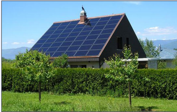
Solar Photovoltaic (PV)
