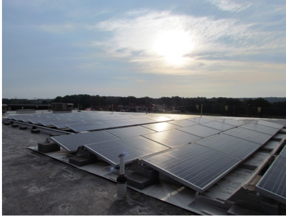
Figure 1 - 10 kW solar system installed as part of the Solar One Pilot Program. Photo courtesy of Columbia Water and Light
