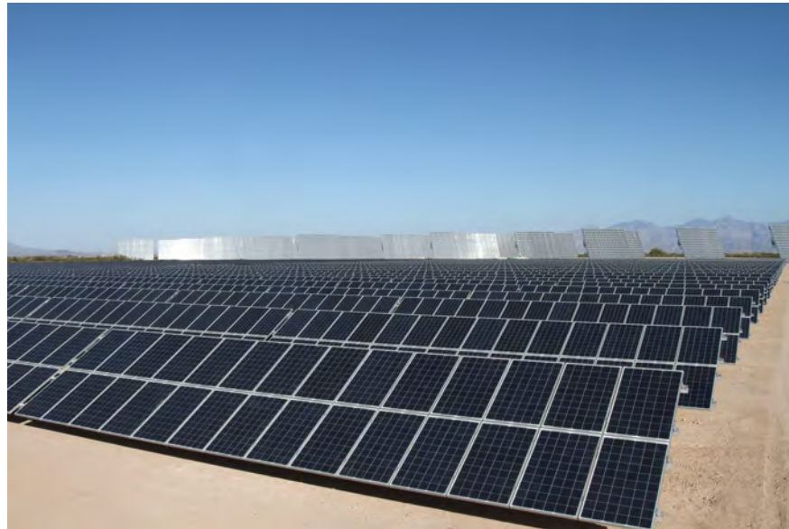
One of Bright Tucson's community solar arrays. Photo courtesy of TEP.
