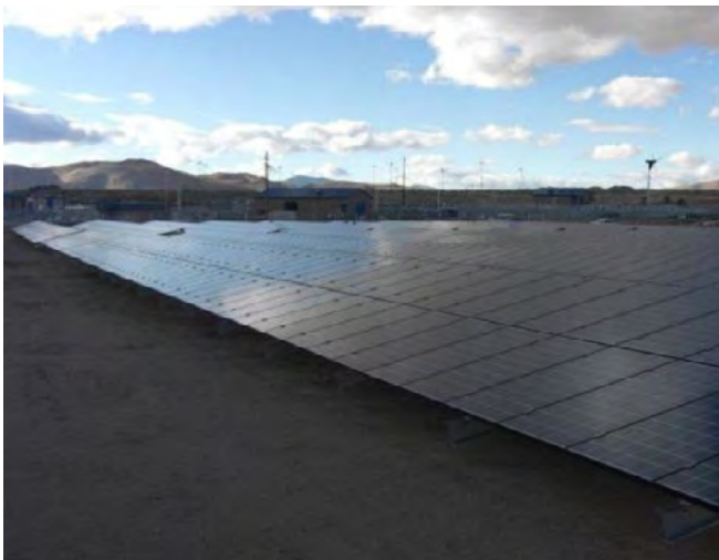
Stead Waste Water Treatment Facility, Reno, NV 6
