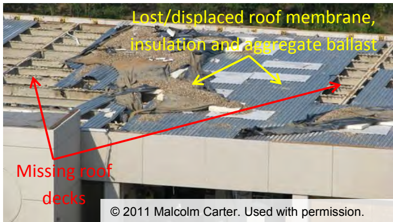
Figure 3–25. Roof of Oncology Clinic Building: missing steel deck panels, gypsum board, rigid insulation, membrane, and aggregate ballast.
