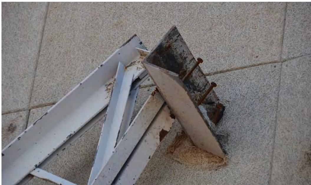
Figure 3–59. Seat angle welded to end of bow–string roof truss and embedded into top of tilt–up panel got disconnected. Note missing vertical headed studs (4, each 10 in. long), which appeared to have been sheared off from the angle. The three horizontal studs remained connected to the seat angle but pulled out from the concrete.
