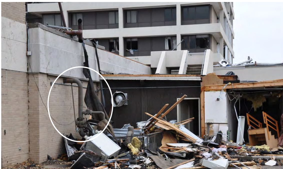
Figure 3–132. High–pressure gas reducer valve at SJRMC that was damaged and leaked.
