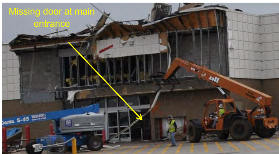
Figure 3–39. Missing door and glass panels and damage to signage at south entrance on west wall (envelope failure allowing air infiltration to the interior and causing increased wind uplift).
