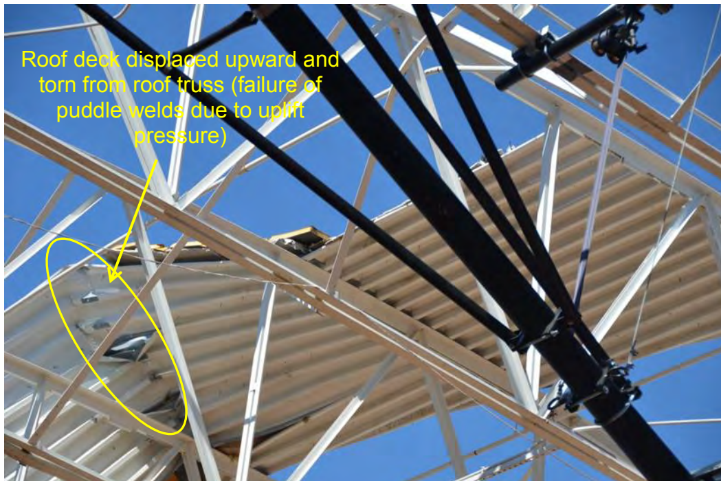
Figure 3–57. Disconnection of steel roof deck of Gymnasium due to failure of puddle welds due to uplift pressure.
