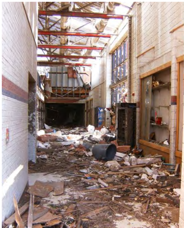
Figure 3–68. Damage and debris in an interior hallway of Joplin High School.
