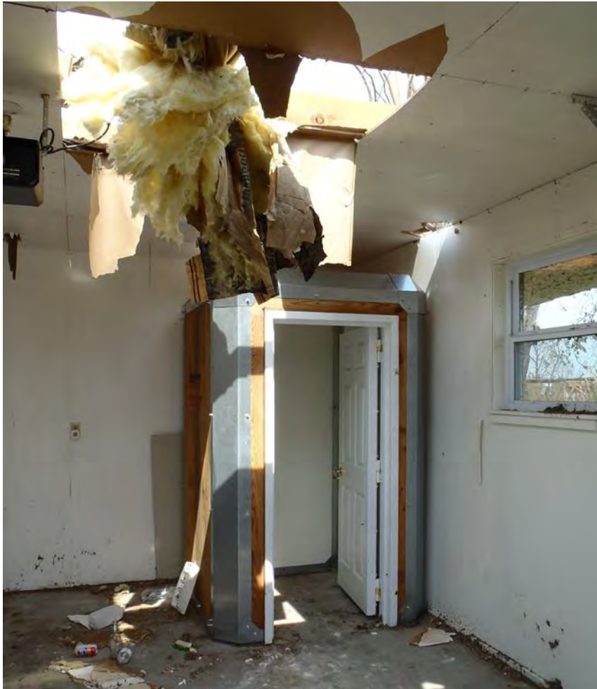
Figure 3–129. Above-ground Kevlar storm shelter bolted to concrete garage floor in residence that was damaged during the tornado.
