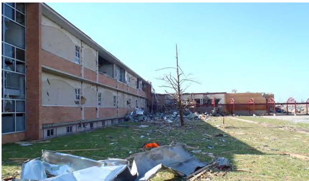
Figure 3–67. View from the exterior showing damage to the envelope of one of the RC frame buildings (west building) of Joplin High School.
