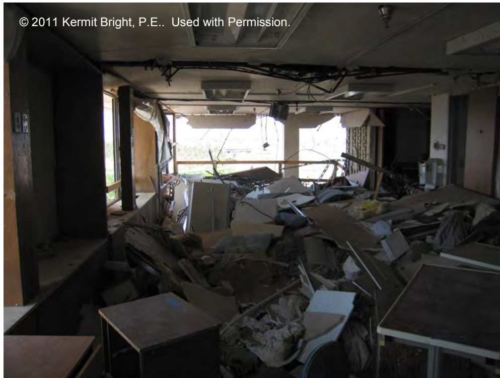
Figure 3–13. Typical damage to the interior of West Tower.
