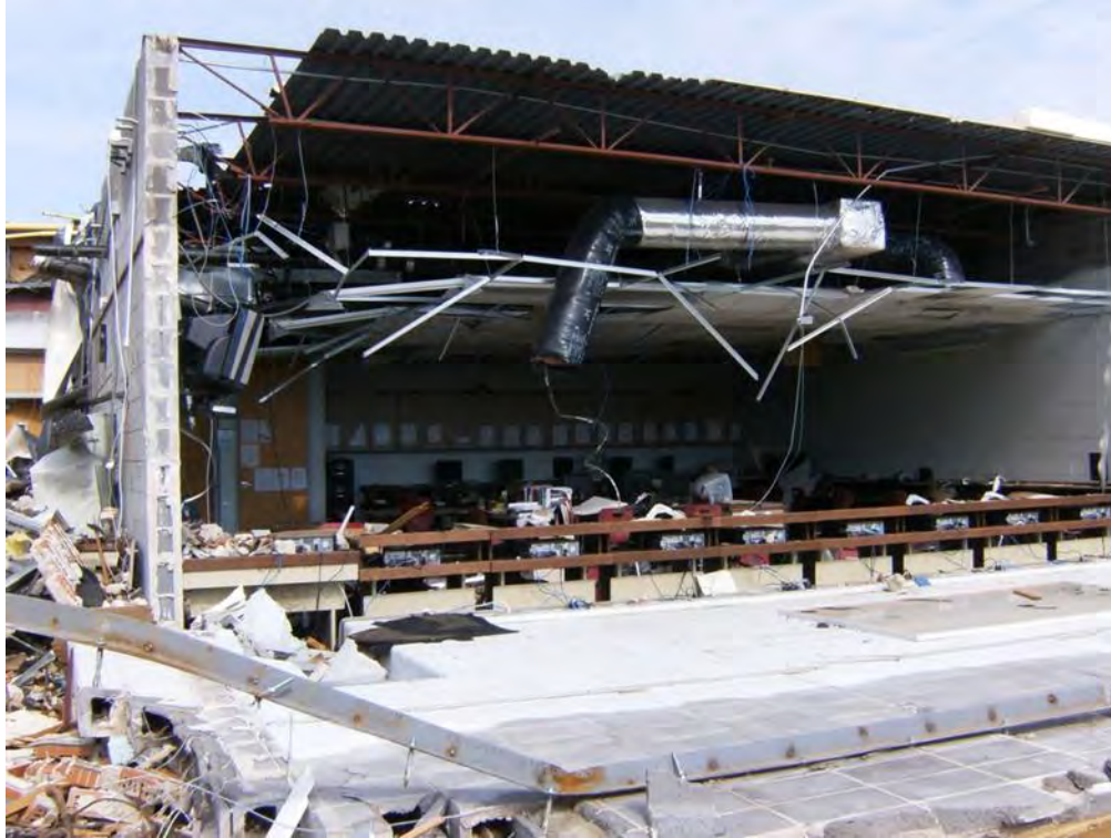
Figure 3–72. Collapse of CMU wall due to loss of lateral roof bracing.
