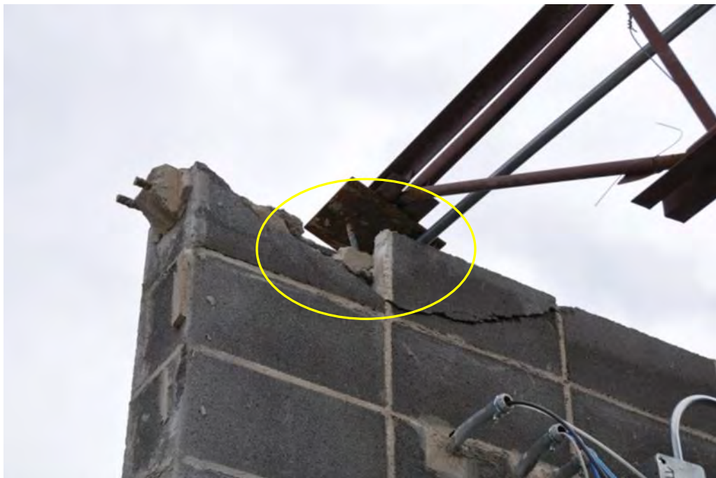
Figure 3–71. Failure of joist-to-CMU wall connection due to uplift.
