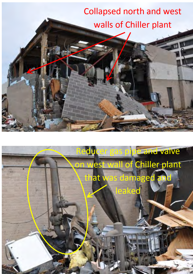
Figure 3–23. Views of damage sustained at the Chiller Plant.
