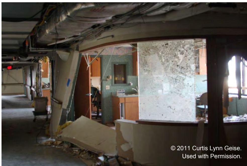
Figure 4-36. Damage to the interior of SJRM.
