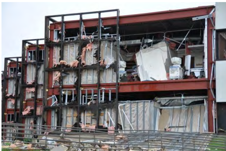
Figure 3–32. Collapse of an entire brick veneer curtain wall and the supporting aluminum stud frame on the south-facing wall of Physician’s Office Building.
