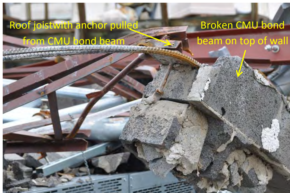
Figure 3–22. Failure details at Emergency Generator Building.
