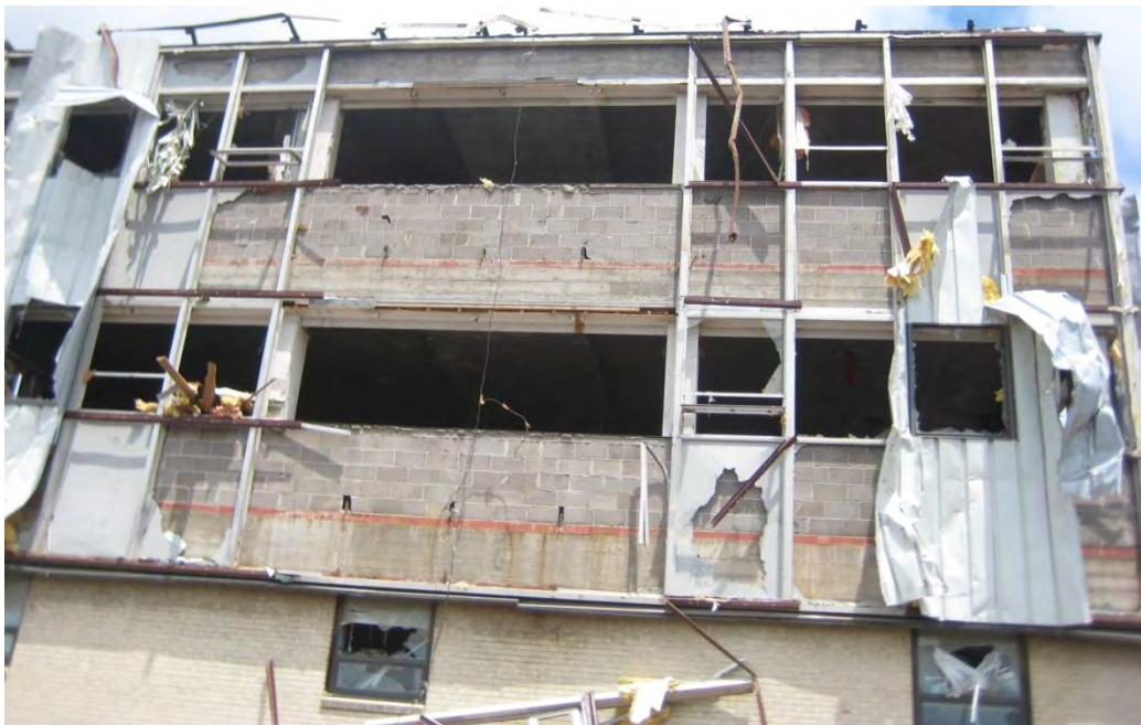
Figure 3–89. Typical damage to the Ozark Center building envelope (broken window glazing, missing window frames, and torn exterior steel panels).
