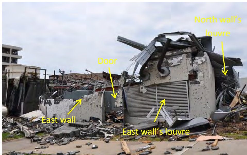
Figure 3–21. East side of Emergency Generator Building. Note eastward direction of failure on east wall (CMU wall falling outward, door opened, louver pushed outward). Also note louver on north wall pushed outward, consistent with direction of maximum westerly wind and indicative of high internal pressure.
