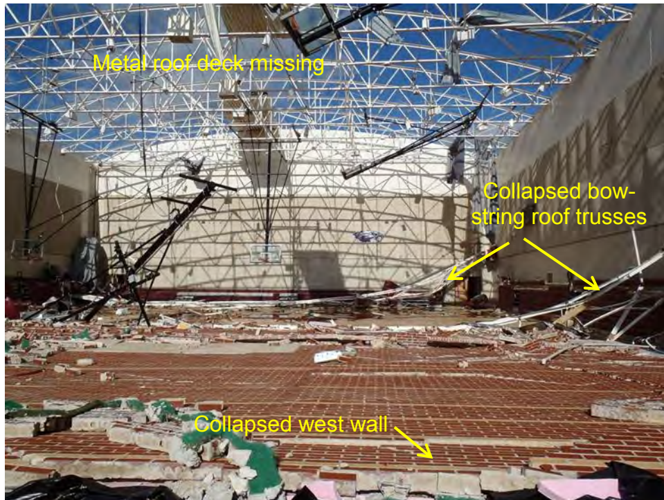
Figure 3–58. Collapsed bow–string roof trusses and collapsed west wall tilt–up panels in the interior of the Gymnasium.
