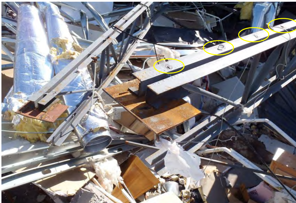
Figure 3–62. In wreckage of Auditorium, missing roof deck from top of joist—only puddle-weld marks remained.
