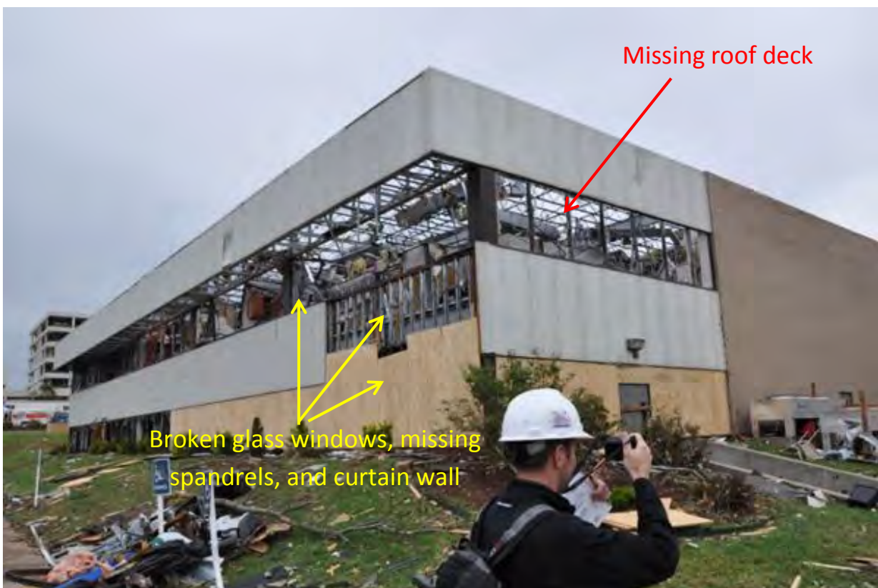
Figure 3–28. View of damage to envelope of Medical Office Building 1.
