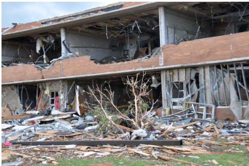
Figure 3–66. View from the exterior showing damage to the envelope of one of the RC frame buildings (east building) of Joplin High School.
