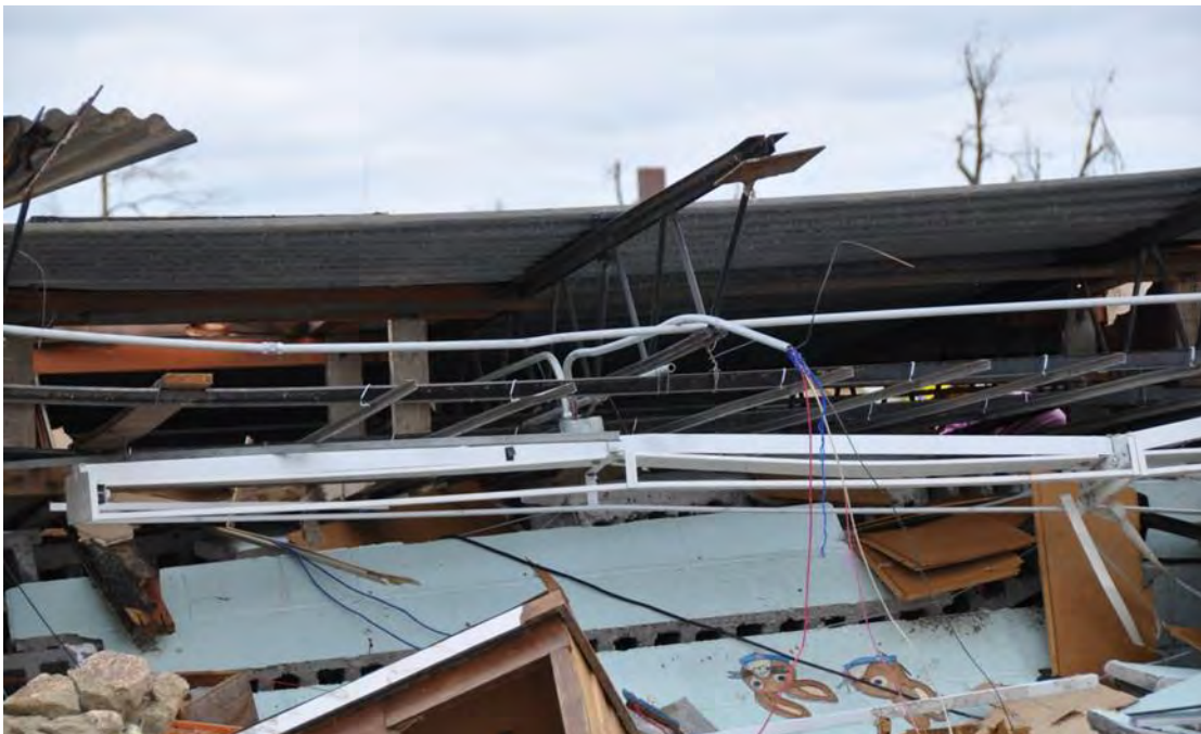
Figure 3–82. Section of building at St. Mary’s Catholic Elementary school with complete loss of the steel roof system.
