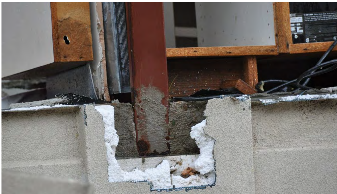
Figure 3–100. Close up view of the Ramesh Shah Ophthalmology Center showing connection between the pre-engineered steel frame with the concrete wall below
