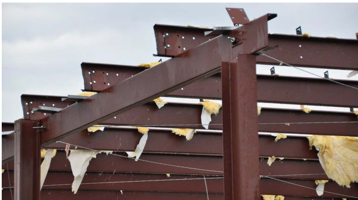
Figure 3–99. Close up view of the Ramesh Shah Ophthalmology Center showing connections and cable bracing of the pre–engineered steel frames
