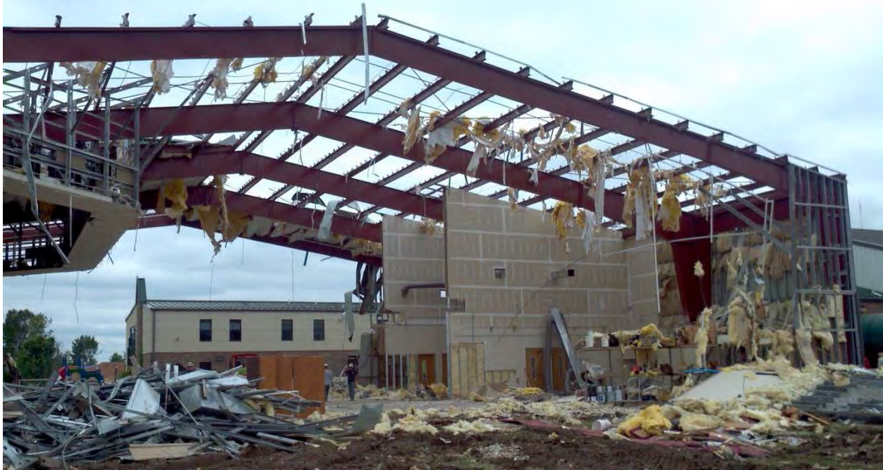
Figure 3–92. View from east of the damaged, pre–engineered steel Mass Hall building of St. Paul’s United Methodist Church.
