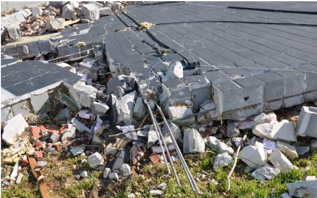
Figure 3–63. Collapse due to overturning (outward) of east perimeter Joplin East Middle School Auditorium wall after loss of roof diaphragm.
