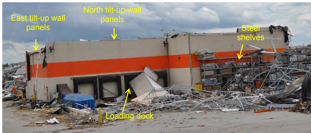
Figure 3–50. Ten tilt-up panels in the northeast corner remained standing. Seven of these 10 panels had positive connections to the footing and thus some degree of restraint against rotation. The other three uncollapsed panels had friction-only connections to the footing but appeared to have been supported against falling outward by steel shelving on the exterior side (Garden Center).
