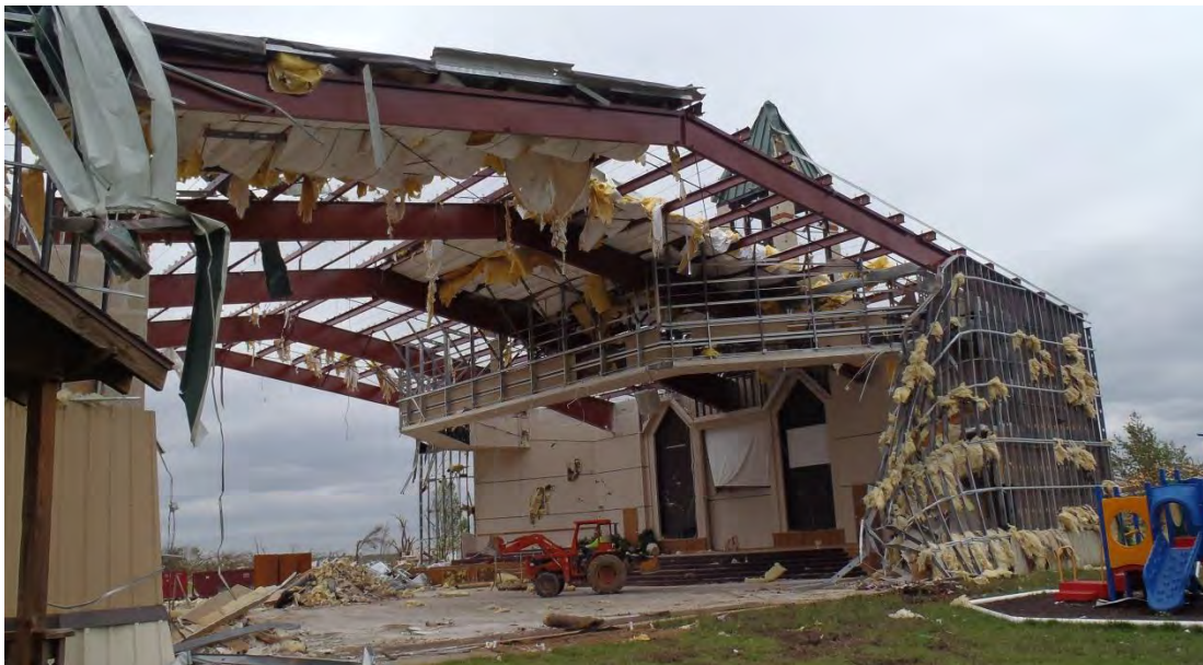
Figure 3–94. Damage to envelope of St. Paul's United Methodist Church.
