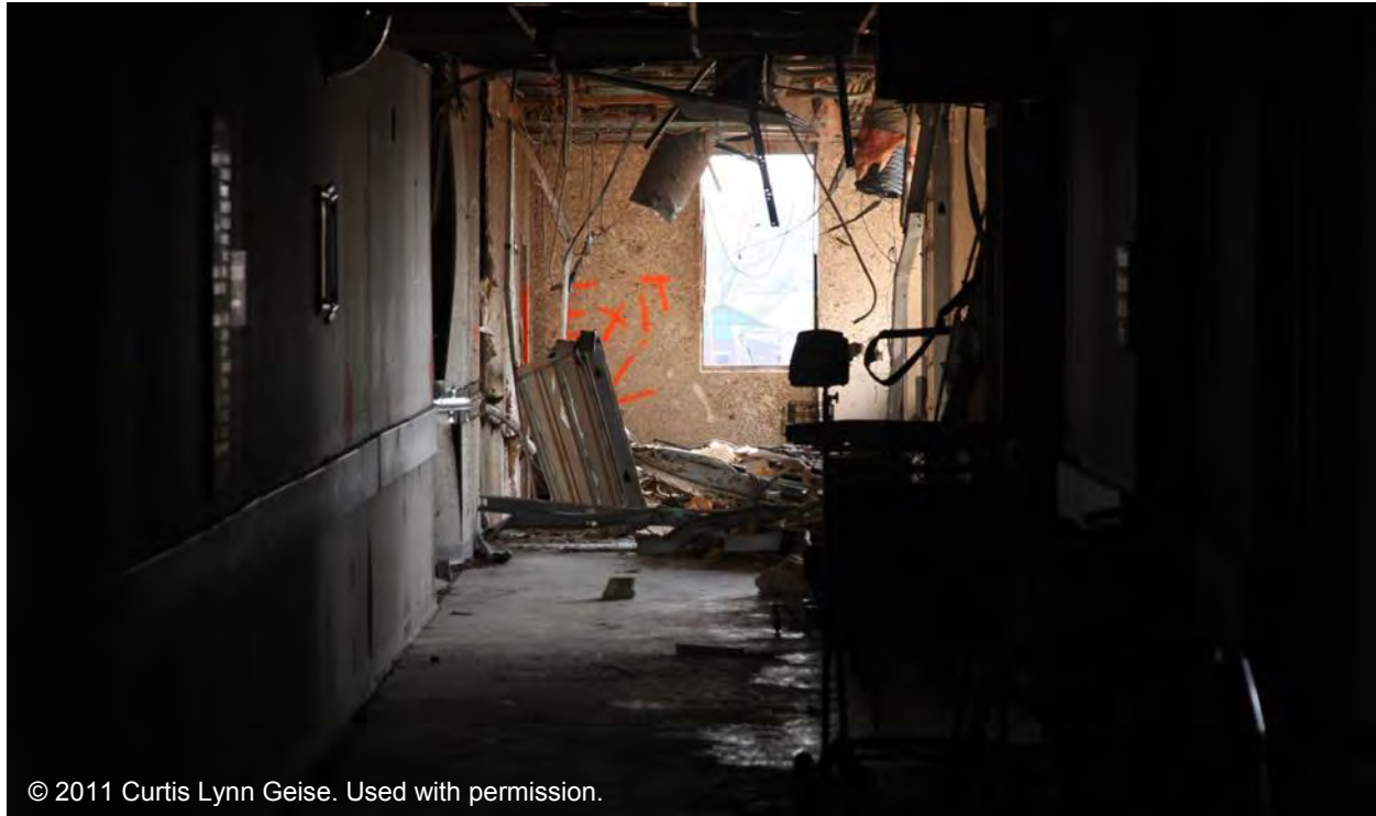
Figure 3–126. View of a typical hallway with damaged interior (ceiling, walls, and debris); hallways were used as designated refuge areas in SJRMC’s East and West Towers.
