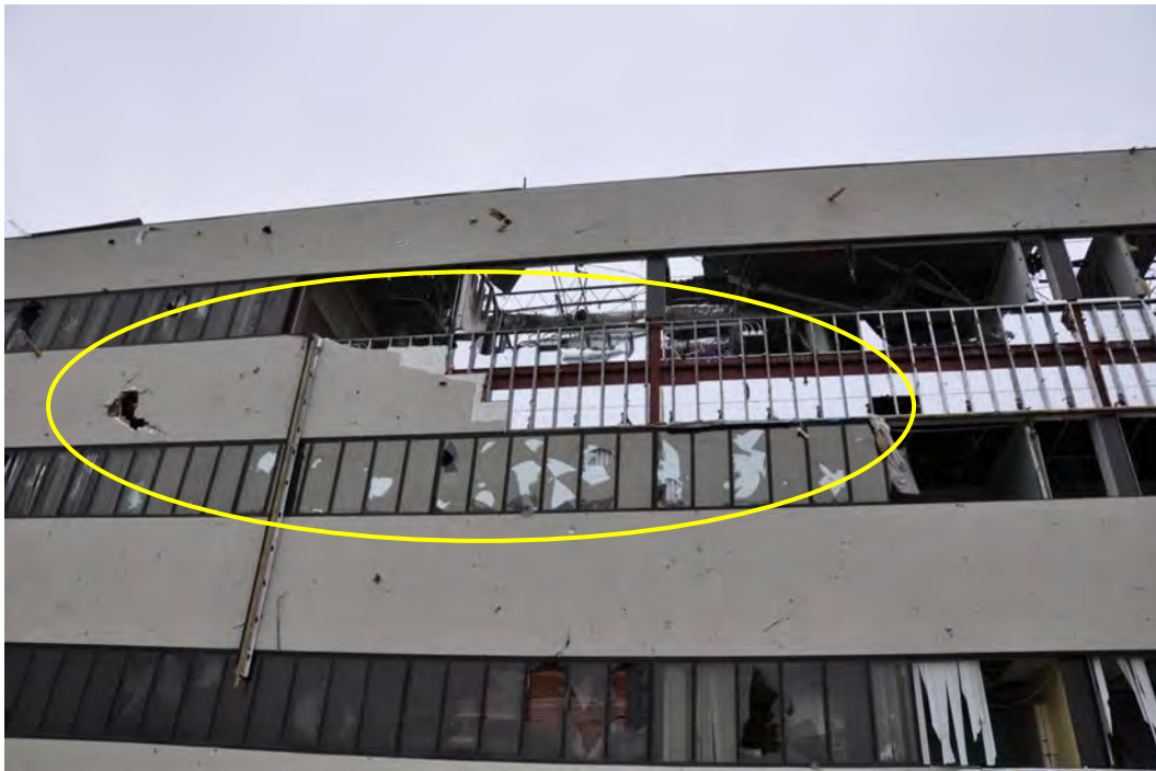
Figure 3–30. Evidence of debris impact causing breakage of windows at Medical Office Building 2.
