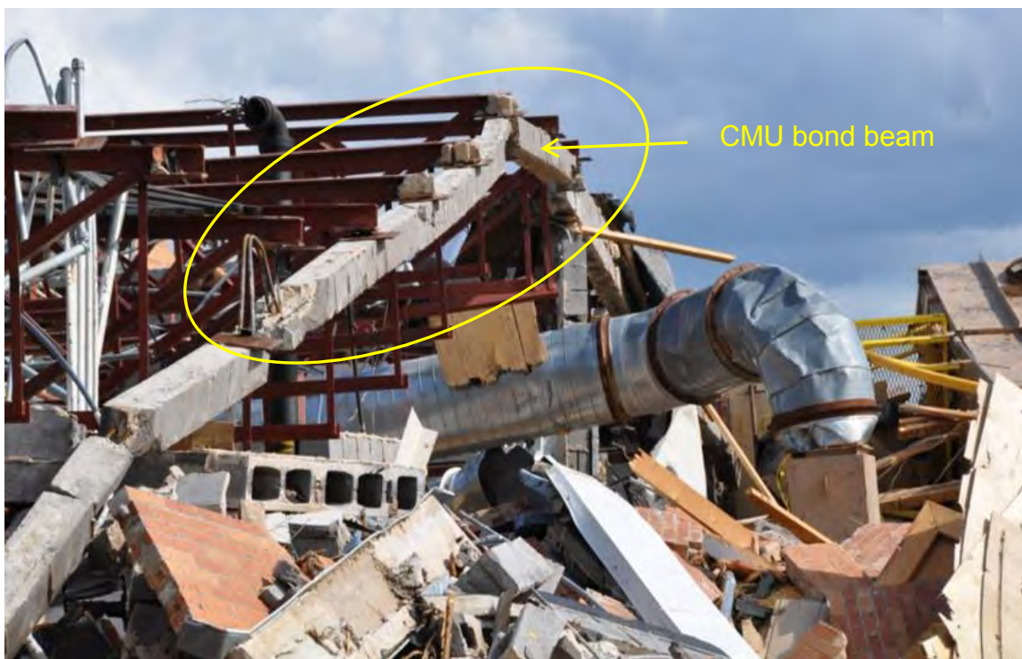
Figure 3–77. Steel roof joists, with missing roof decks, remained connected to CMU bond beam. Bond beam remained continuous, but was disconnected from the CMU walls along the bond line between the two CMU courses at the top of the wall.
