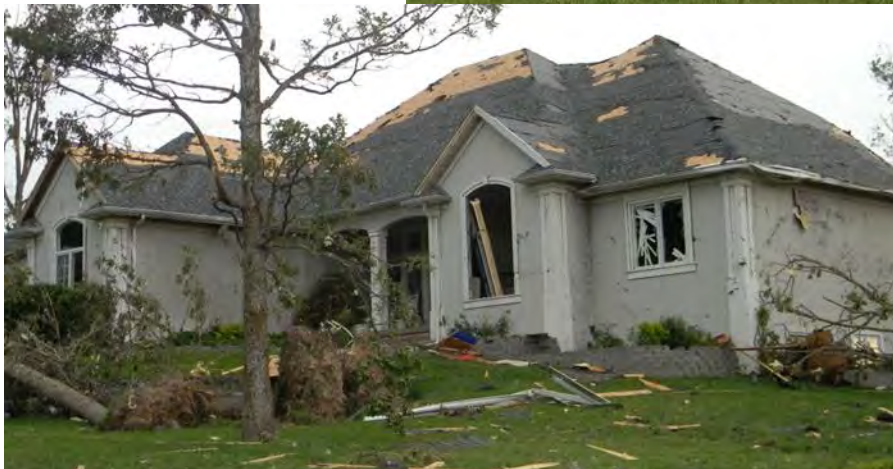
Figure 3-118. Typical damage to residential dwelling envelope.
