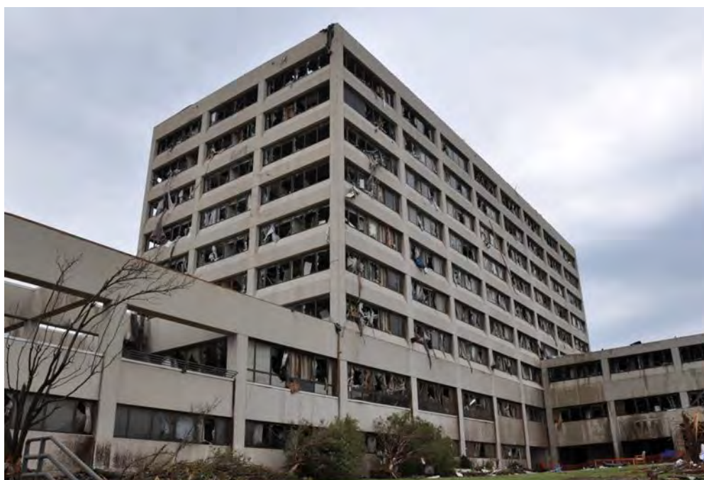
Figure 3–15. View from southeast of East Tower showing that most windows on south and east sides of building have broken.
