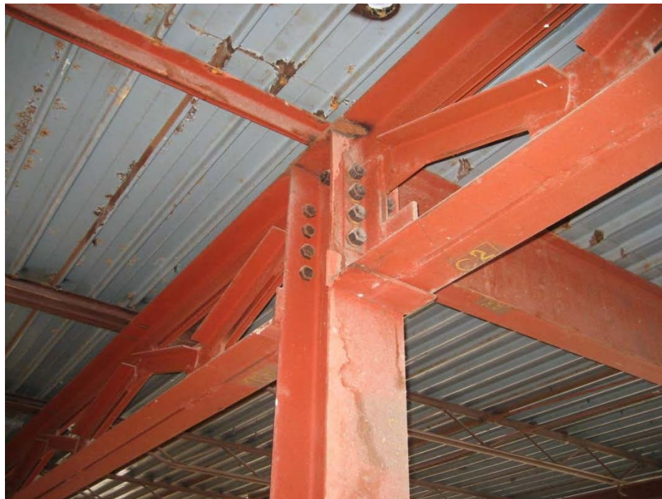
Figure 3–87. Interior view of the physical education section of the Ozark Center showing structural system with roof truss–column moment connection and open–web roof joist and wide–rib steel roof deck.
