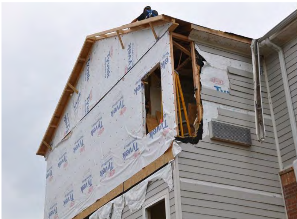
Figure 3–112. Damage to the building envelope of the Mercy Village Apartments.
