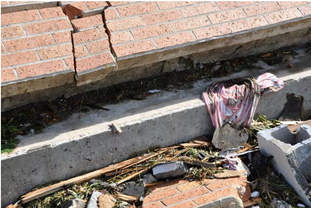
Figure 3–79. Perimeter CMU wall that collapsed after loss of roof lateral bracing (note lack of reinforcing dowels connecting wall to concrete footing).
