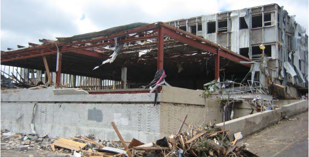
Figure 3–88. Significant damage to the envelope and minor damage to the MWFRS of the physical education section of the Ozark Center building, including (1) loss of part of steel roof decks, (2) loss of all insulating windows and steel frames on all wind-exposed sides, and (3) deformation of steel beam (likely due to debris impact).
