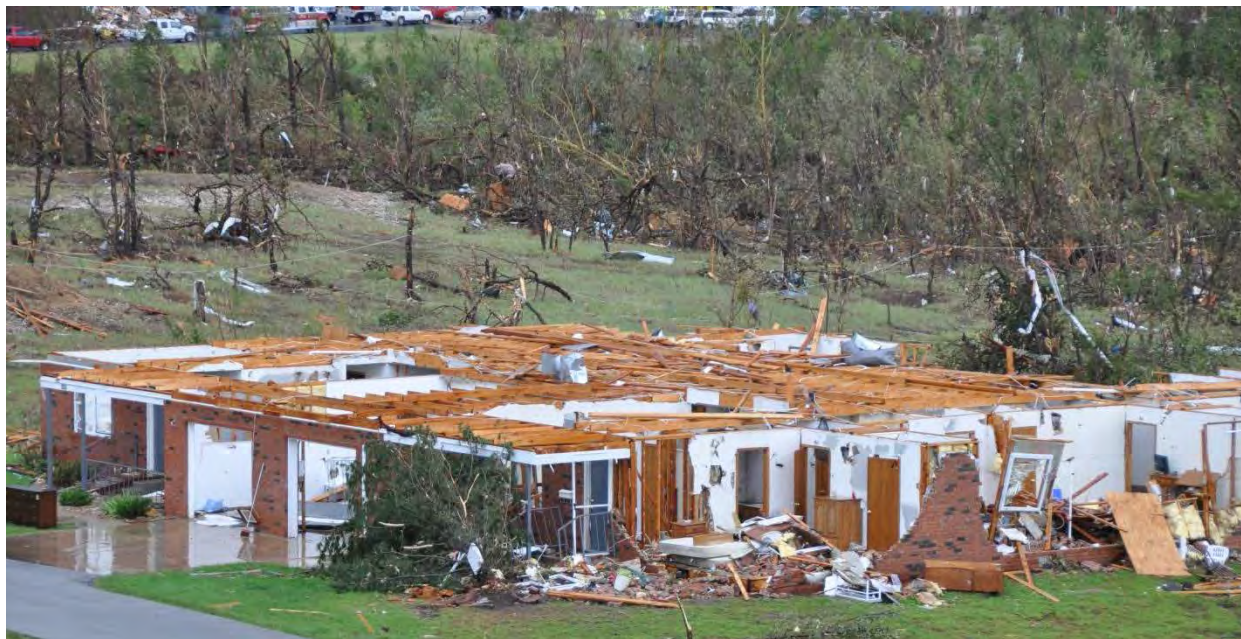
Figure 3–115. Disconnection and loss of entire roof system.
