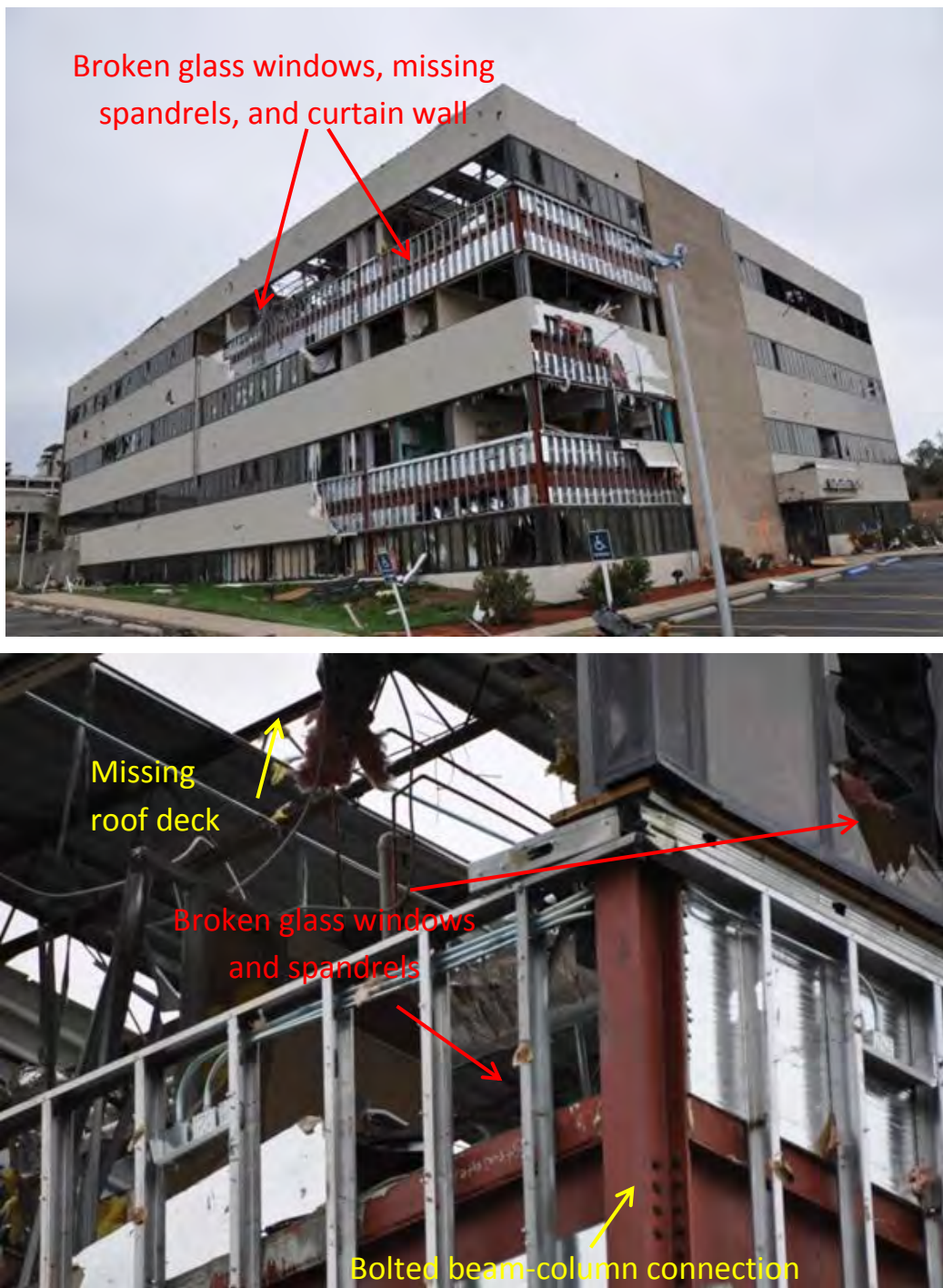
Figure 3–29. Views of (top) damage to envelope of Medical Office Building 2 and (bottom) portion of the steel frame system (bolted beam–column connection).
