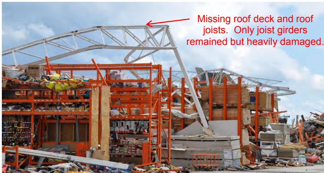
Figure 3–51. Damaged joist girders and interior columns. Note the complete loss of the roof system that was connected to the girders.
