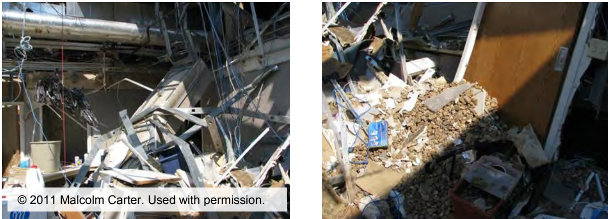
Figure 3–27. In Oncology Clinic Building, interior damage to ductwork, electrical wiring, suspended ceiling, interior partition/metal stud wall, furniture. Note the aggregate from roof in the interior.
