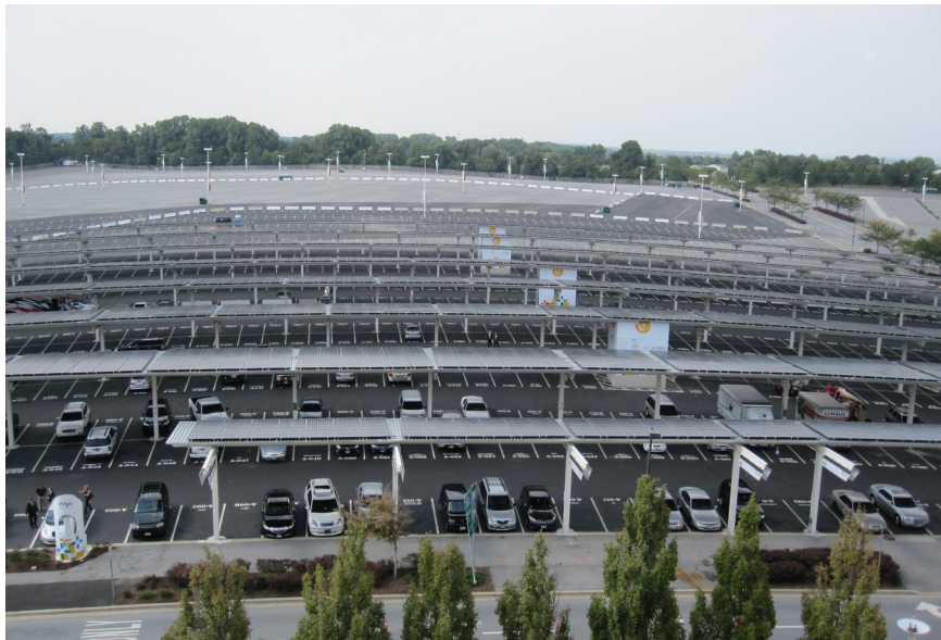
Solar Panels at FedEx Field.
