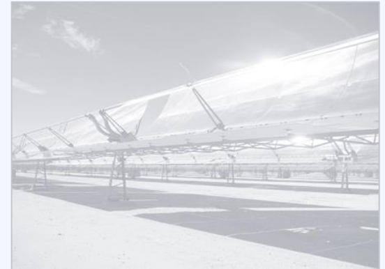
Concentrated Solar Power
