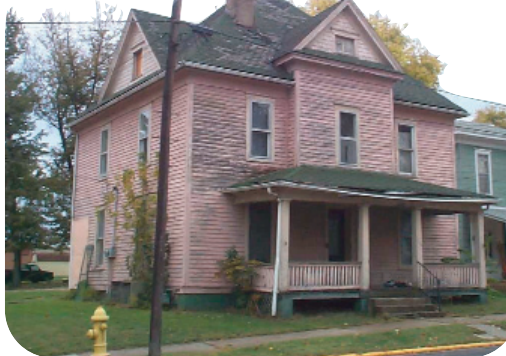
A dilapidated multi-family residence in Jacksonville before renovation
