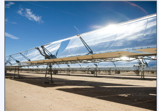
Concentrated Solar Power
