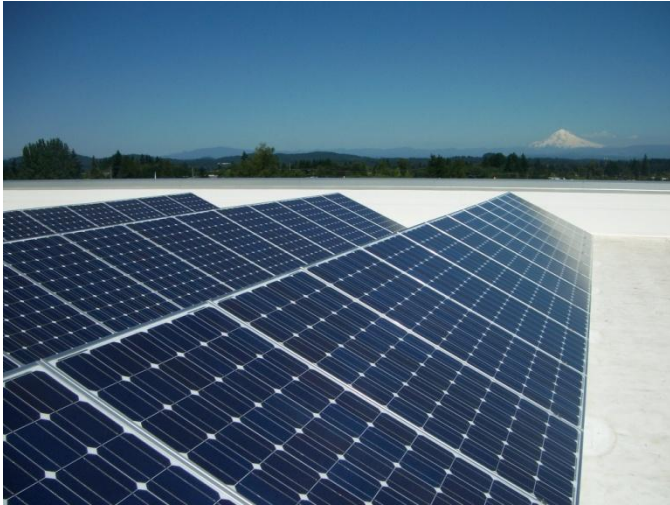
Clackamas County has a 67kw array on its Development Services Building, seen here with Mt. Hood in the background.
