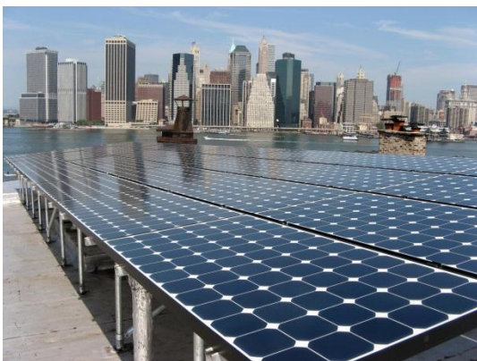
Rooftop Solar in New York Photo courtesy of Aeon Solar
