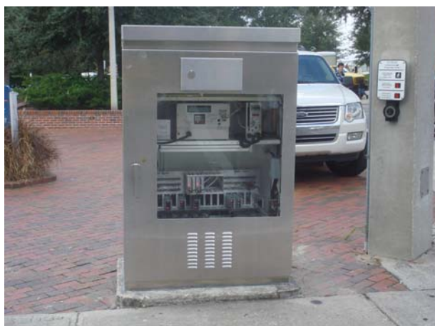
Traffic Signal Cabinet with front door window.
