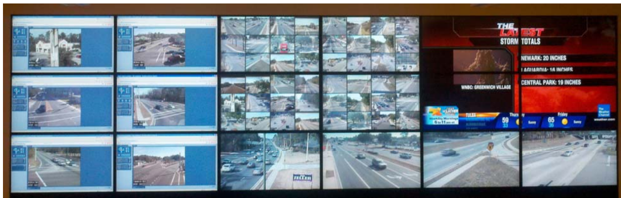
Video Wall in Traffic Management Center – 21' x 7'
