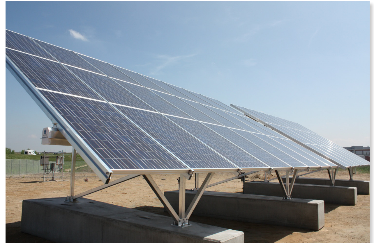
United Power's Sol Partners Installation, Colorado
