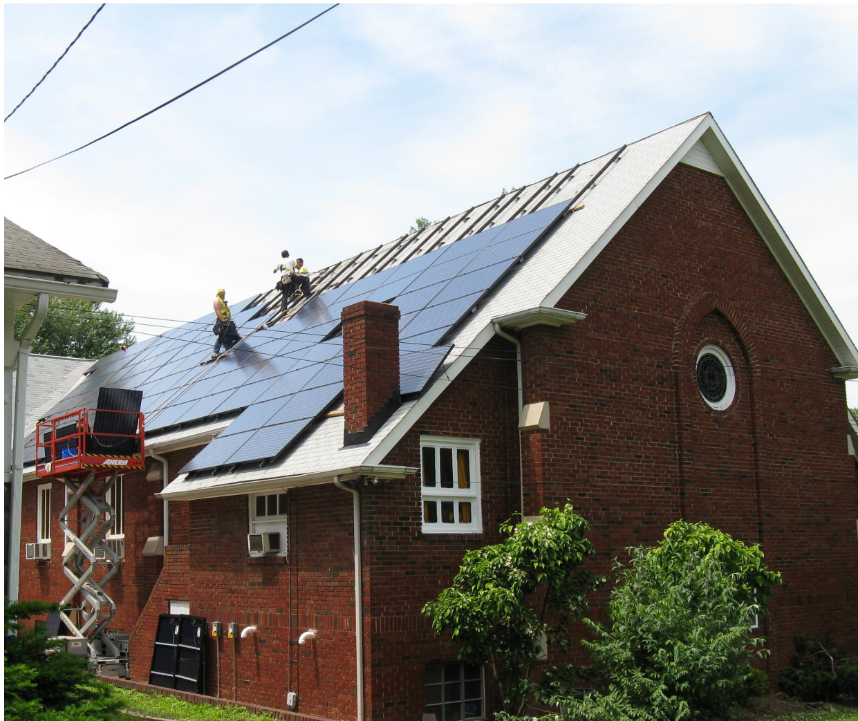
Panels on a Steep Roof, University Park, Maryland
