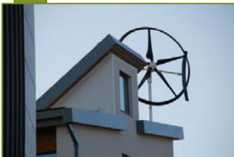
Building mounted wind turbine
