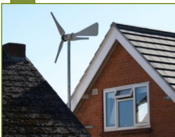
Wind energy conversion system
