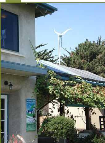
Wind energy conversion system
