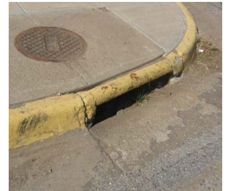
These images represent the current stormwater infrastructure that could be enhanced by green solutions.
