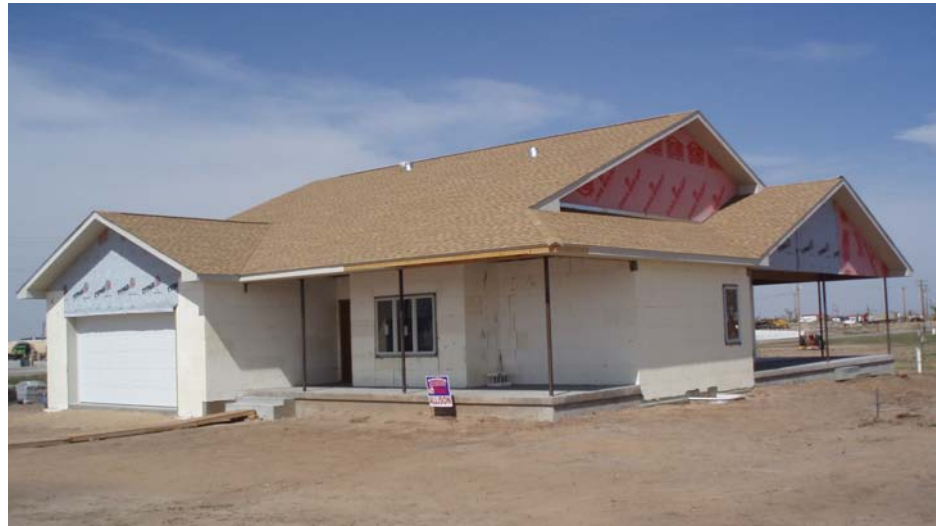
The Alison Home in Greensburg is built from Insulated Concrete Forms (ICF) and is 58 percent more efficient than residential building codes dictate, it easily meets the recommended residential efficiency target.
