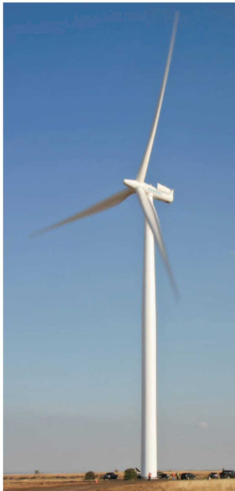
The 2.3-megawatt Siemens wind turbine installed at the National Renewable Energy Laboratory is the centerpiece of a government-industry research partnership between Siemens and the laboratory to study the turbine's performance and aerodynamics.
