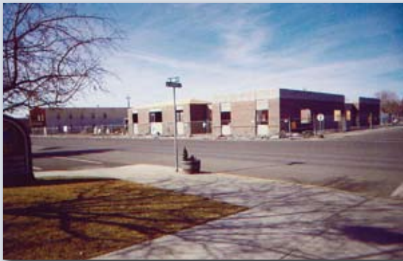
During construction on the new City-County Government Services complex on the same corner
