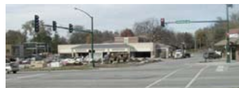
A main Windsor Heights thoroughfare was widened and reconstructed, as part of efforts to revitalize city.
