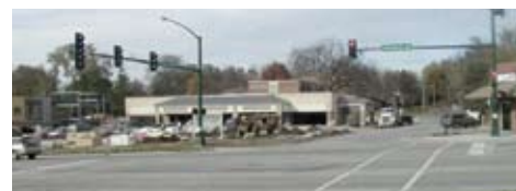
A main Windsor Heights thoroughfare was widened and reconstructed, as part of efforts to revitalize city.
