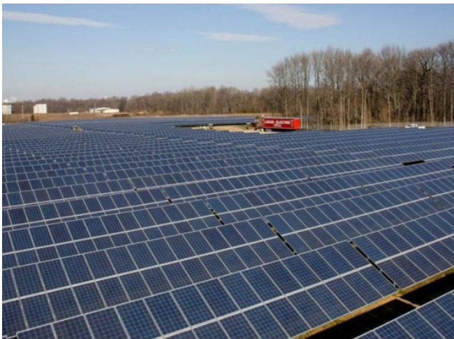
819 KW Solar Array at Barnstable Water Pollution Control Facility
