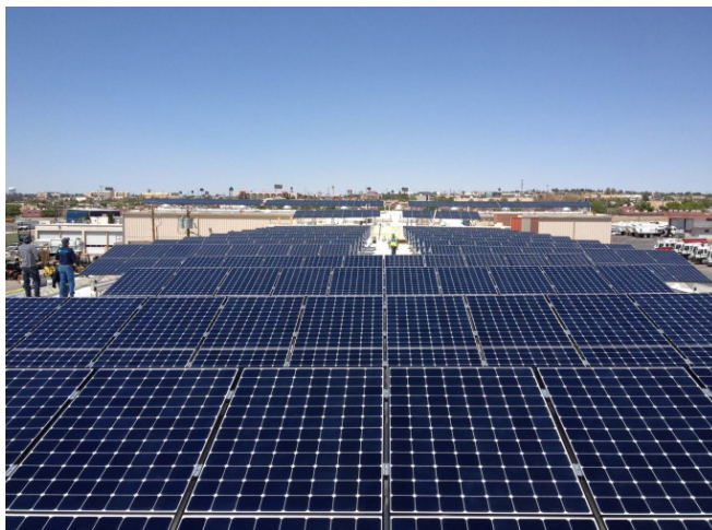
Rooftop solar PV on El Paso Municipal Service Center
