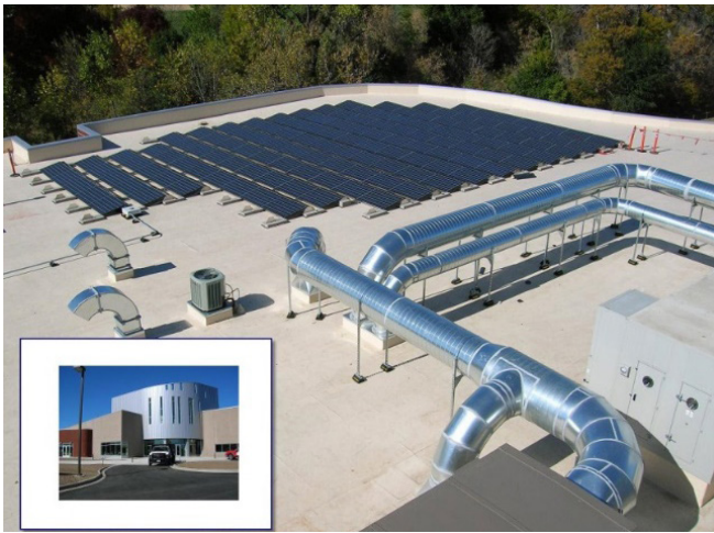
The Fort Collins Museum of Discovery 36 kW PV array
