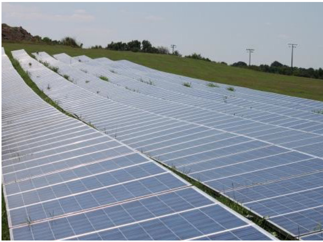
Ground Mounted Solar Array at the Franklin Wastewater Treatment Facility
