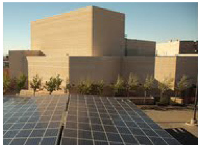
Solar array at Lancaster’s Performing Arts Center
