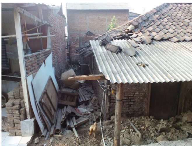
Figure 9. Land subsidence in Tambak Lorok
